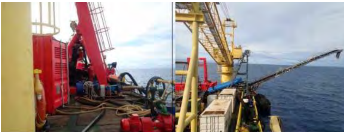
Photo 8. Extraction/siphon pump (left); Flyout conveyor where waste materials will go back to the sea
